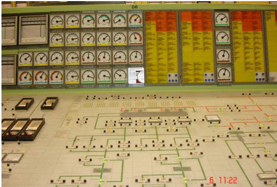
FIG. 33. Conventional indications and status lights in a control room.
