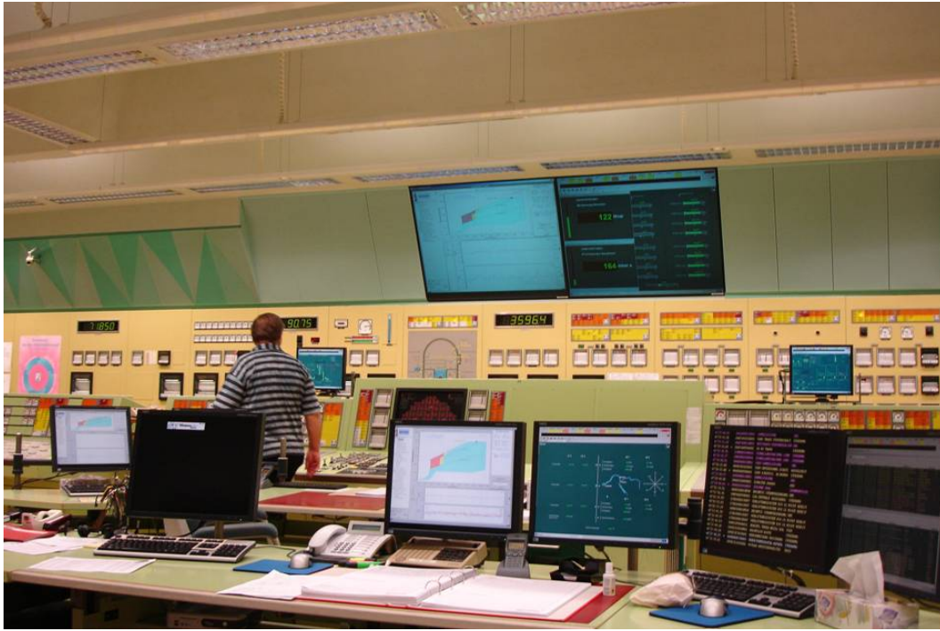
FIG. 39. Computerized workstations and large overview displays along with conventional indications in a hybrid control room.
