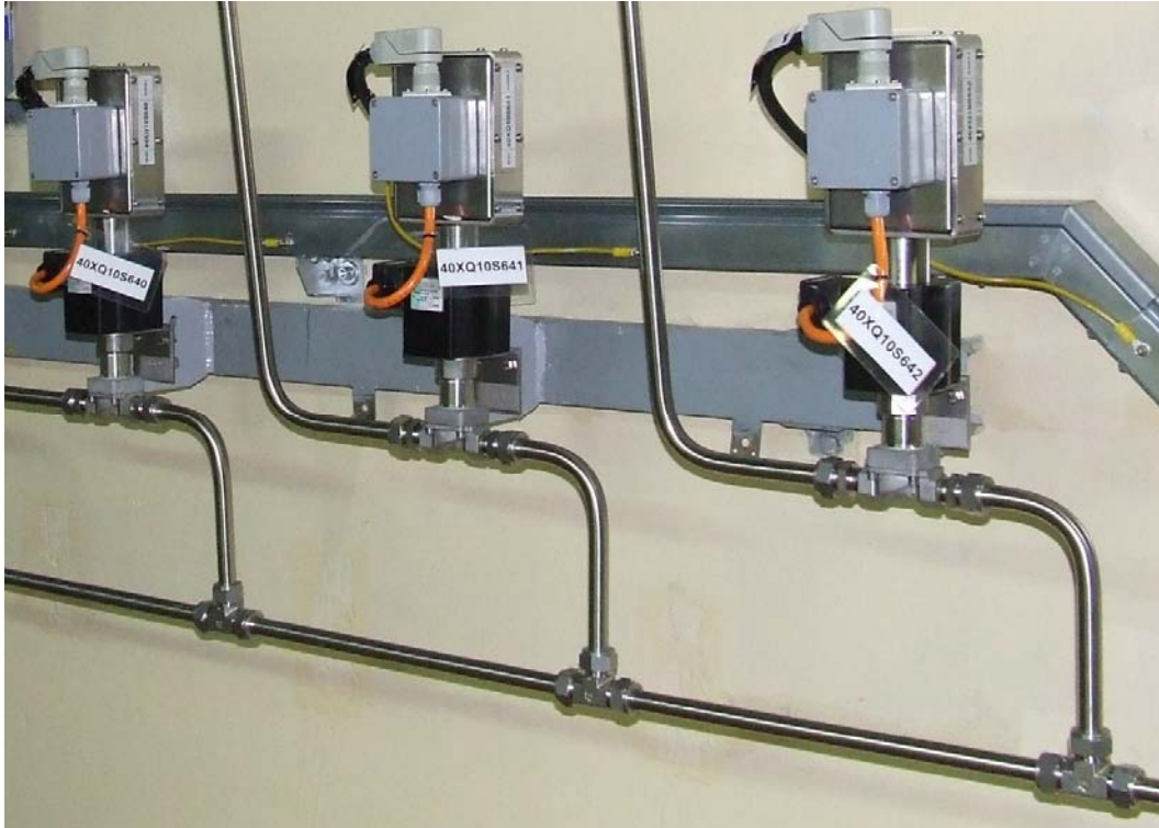
FIG. 16. Solenoid valves controlling air sampling.
