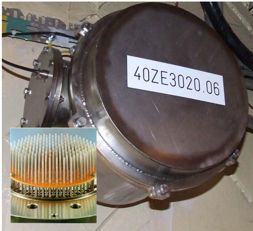
FIG. 21. Containment wall cable penetration (with the internal part in the small photo).
