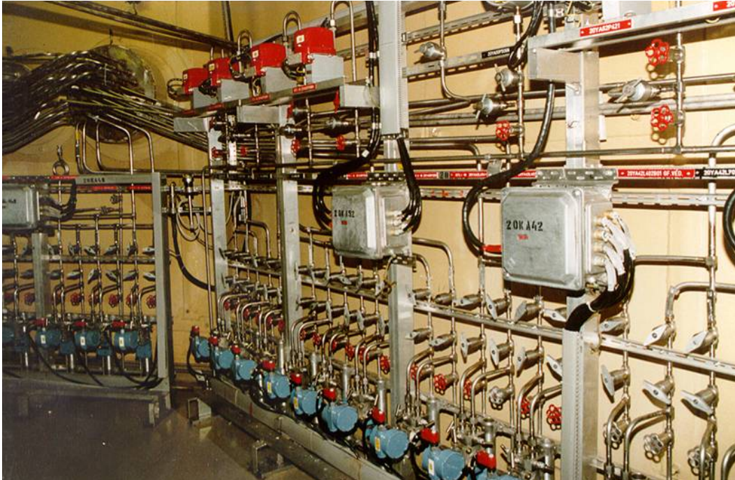
FIG. 10. Instrumentation tubing (impulse lines) in the containment area.
