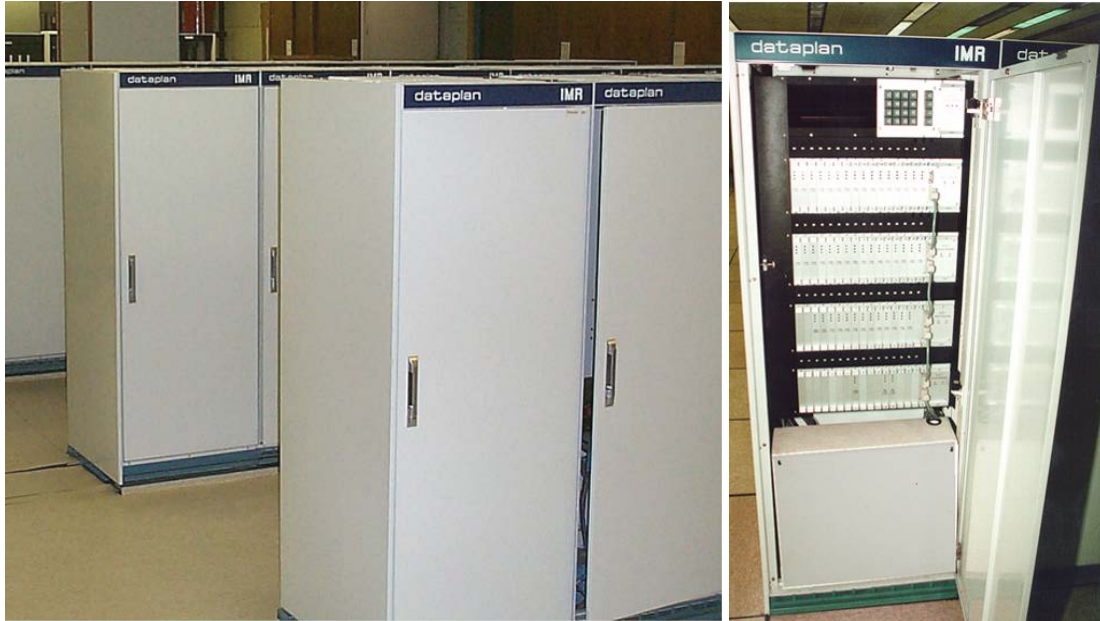
FIG. 23. Centralized data acquisition cabinets.
