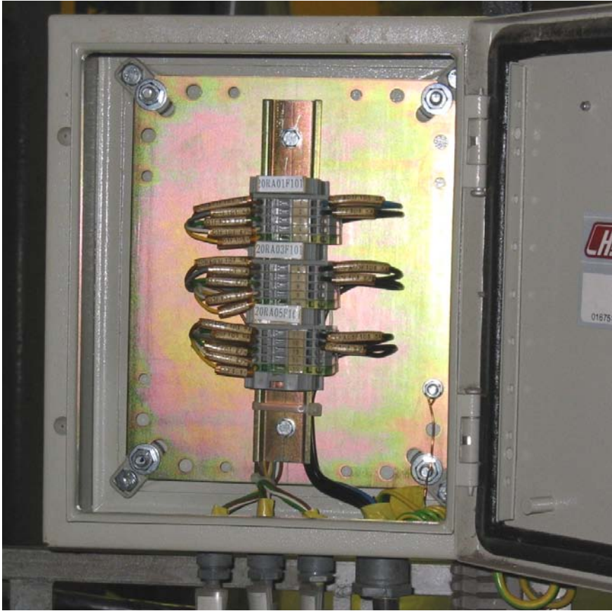
FIG. 20. Junction box with terminal block.
