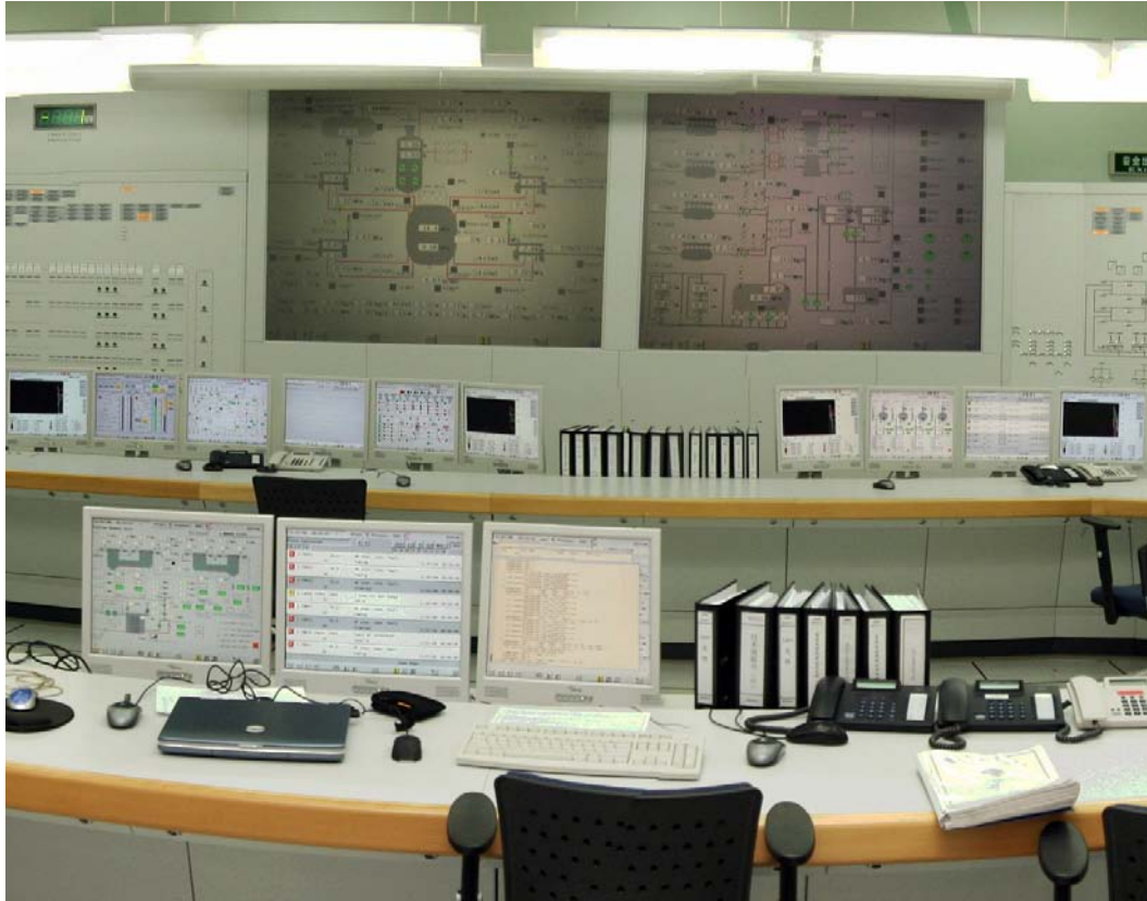
FIG. 36. Large panel displays in a main control room.
