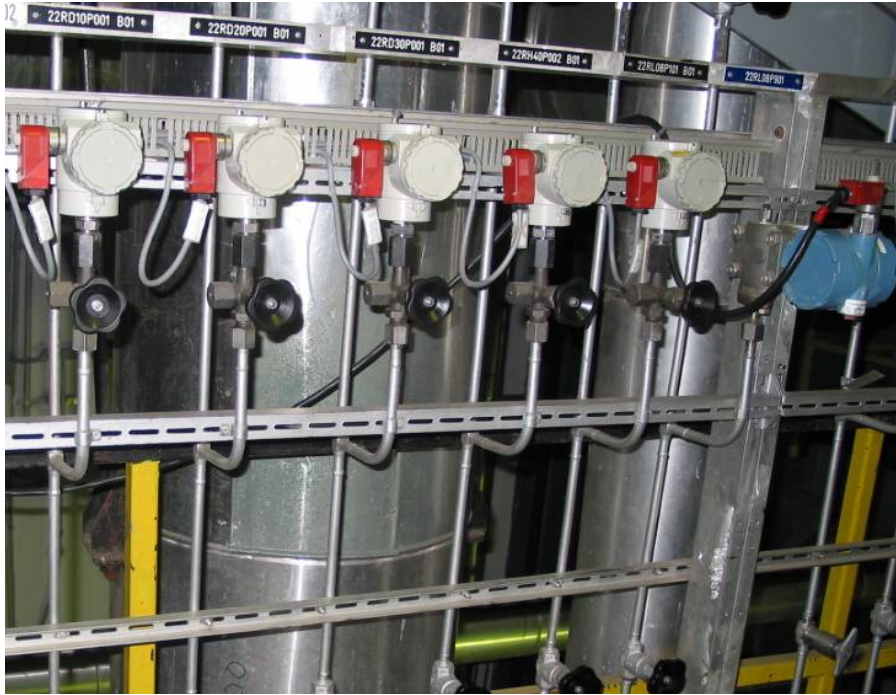
FIG. 7. Pressure transducers installed on a transmitter rack.
